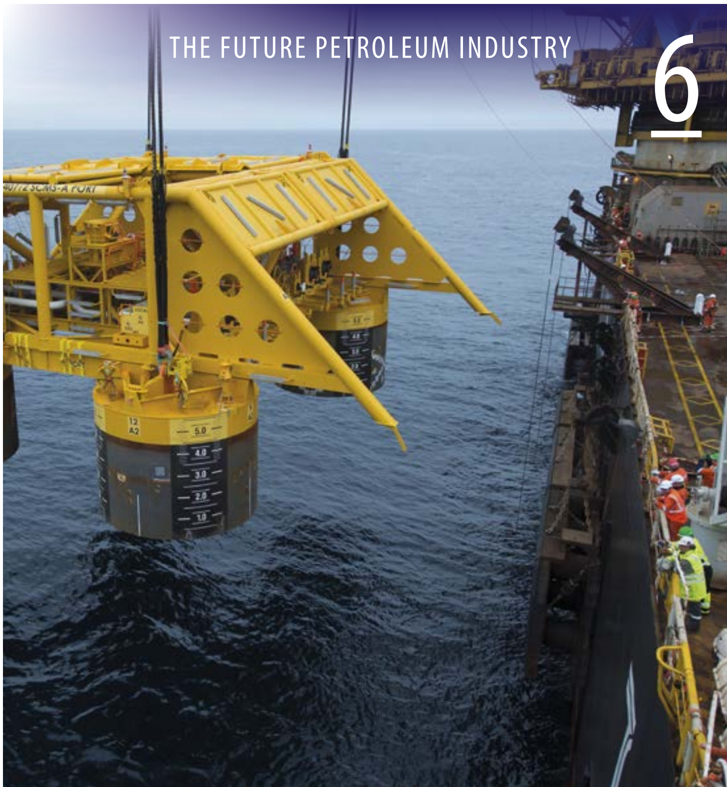
Installation of subsea compression equipment on the Åsgard field in the Norwegian Sea. This is innovative technology that will contribute to a substantial increase in gas and condensate production from the field (Photo: Øyvind Hagen, Statoil)
