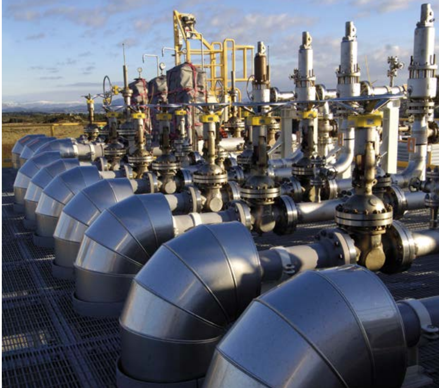
From the Kollsnes gas processing plant in Hordaland County. Gas from a number of fields, including Troll, is processed here (Photo: Øyvind Sætre/Gassco)
