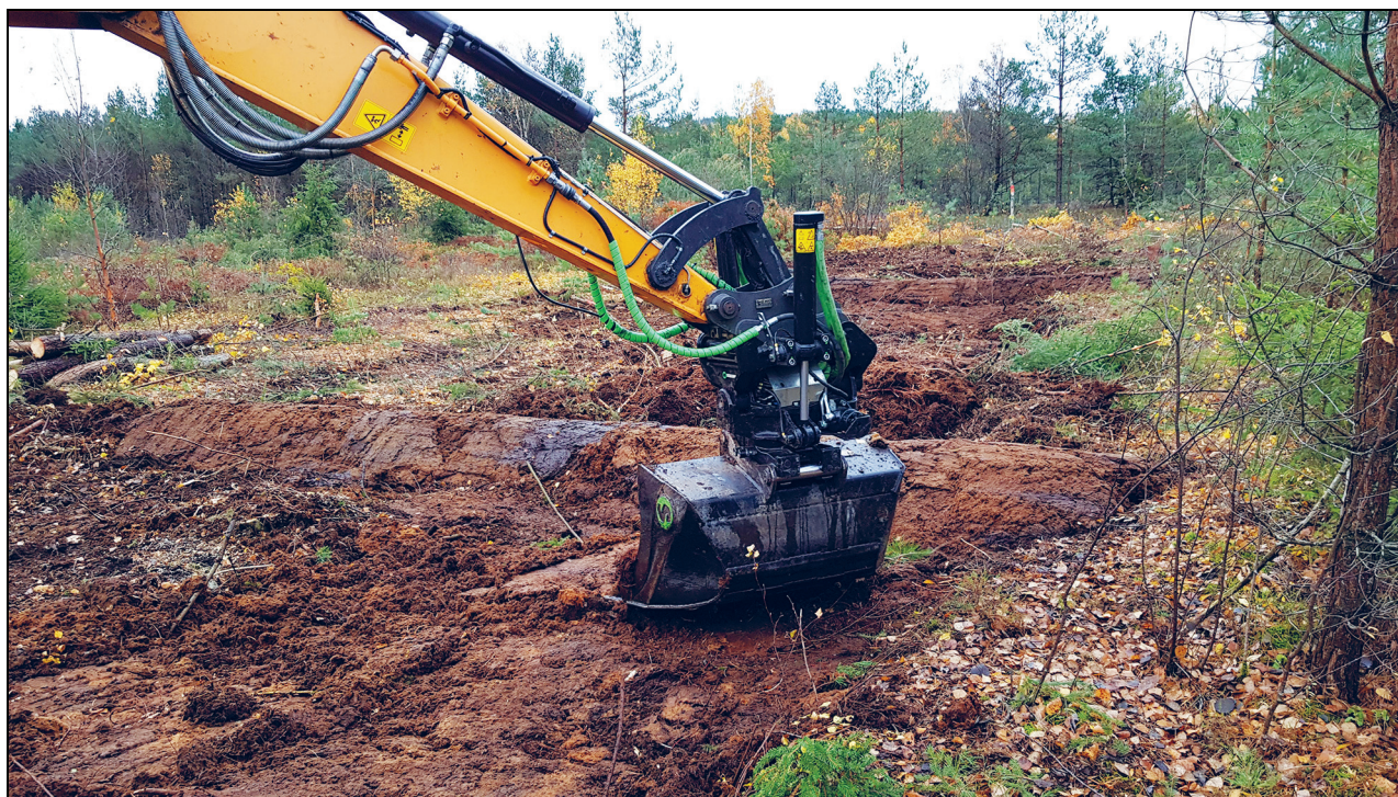
Figure 4.10 During peatland restoration, old drainage ditches are blocked with peat and other material from the site. The surface vegetation in the ditches is removed by the excavator before infilling and then replaced.
