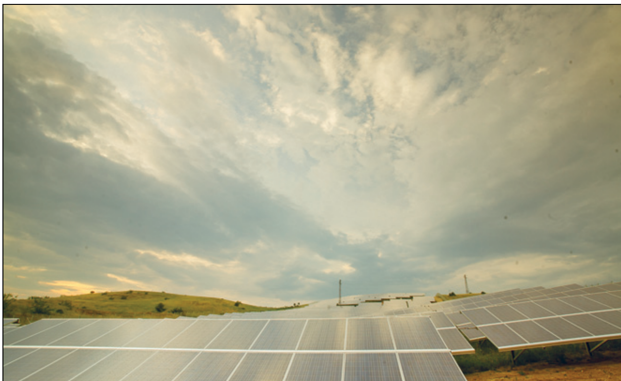
Figure 5.3 The solar energy park Pripechene, in Bulgaria, was established with funding from the EEA and Norway Grants. The project was implemented by Hydroenergy Company Bulgaria in cooperation with Norsk Solkraft AS.
