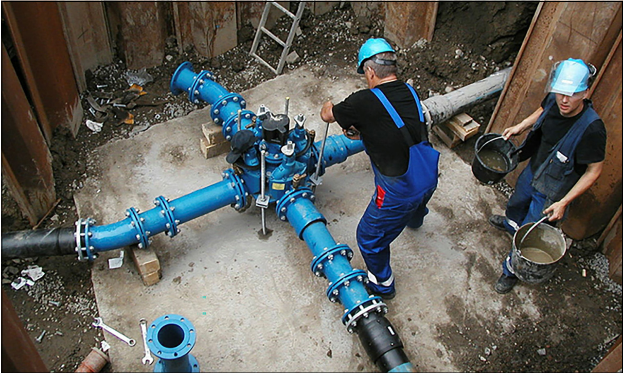
Figure 4.9 Renewal and maintenance of the water supply network is important for safe drinking water.
